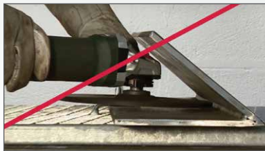
This solution violates safety standards
